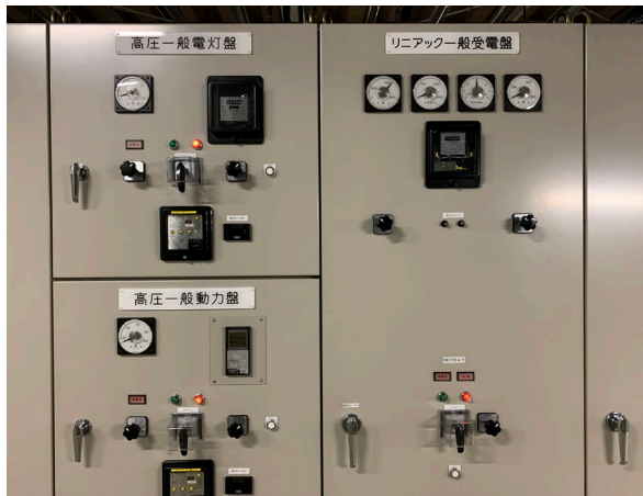
Figure 7: Photo of the high voltage switchgear where the analog indicating meters will be replaced. Replace one of the multiple analog indicating meters installed in the high voltage switchgear with a digital multimeter. By replacing one analog indicating meter with the digital multimeter, multiple values, such as power, power factor, etc., can be monitored simultaneously.
