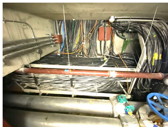
Figure 3: Over many years of operation, a large number of cables have been laid to the radiation area from the control room and computer room, and the resources for cable routes are scarce.
