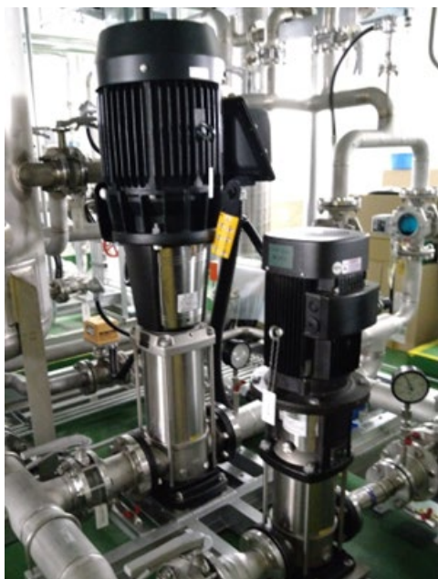
Figure 6: A large water pump for normal operation and small one for standby operation in a night.
