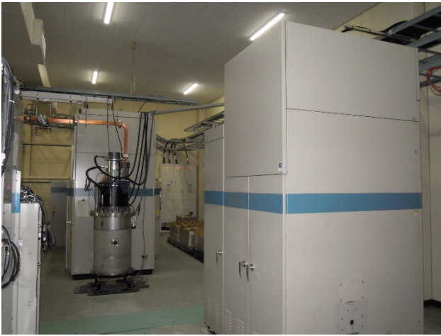
Figure 6: Current status of the planned update site. A housing for a small modulator (right) and a large modulator and a klystron (left).
