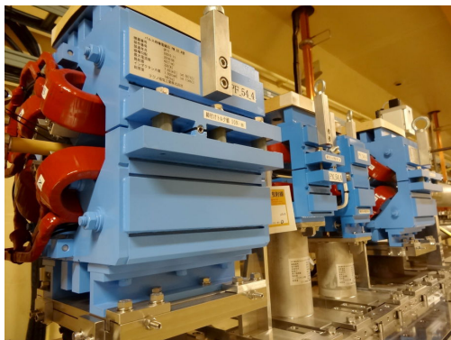
Figure 2: Example of pulsed magnets installed in the linac.
