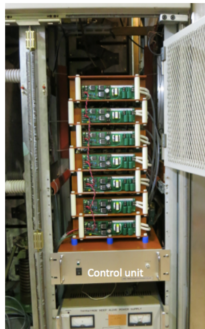
Figure 3: Solid-state thyatron replacement switch installed in modulator.
