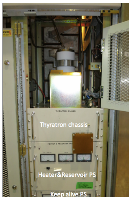
Figure 2: Thyatron switch tube installed in modulator.
