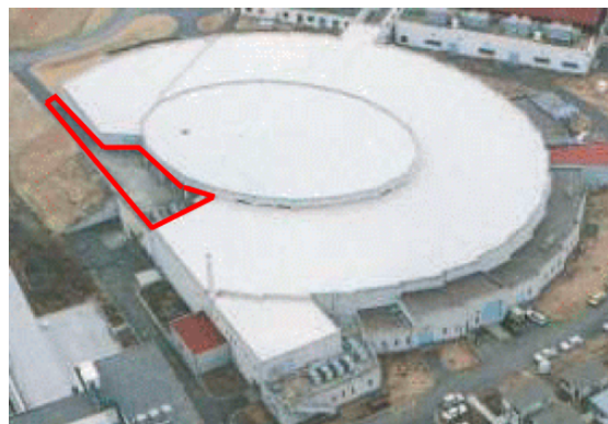
Figure 5: Photograph of the PF Light Source Building. The white roof shows the thermal insulator for suppression of building distortion and the area bordered by a red line is the roof of the injection area with a beam transport line where the thermal insulator is not installed.
