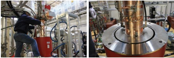
Figure 6: Adjustment of clearance between main klystron and magnet coil.
