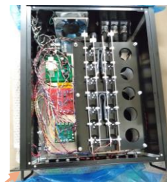
1 mF capacitor x14 in Capacitor chassis
