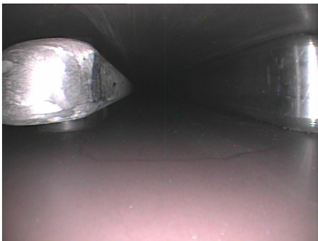
Figure 4: Examples of discharge mark. Upper picture shows the discharge in the insulator and the lower the creep discharge on the surface of the insulator. Both the discharge cases caused burnout of the diode stacks.
